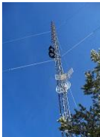
KGLP's Antenna is on this Tower (It's the two black rings.)
