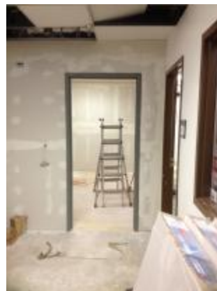
The Work-in-Progress of KGLP's December 2014 renovation, which opened up space for a 2nd studio, and included new paint & carpet.
